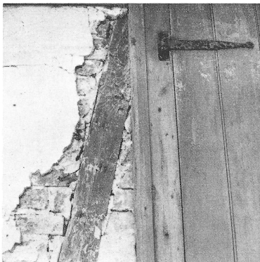
Detail of briquette-entre-poteaux construction, showing a wrought-iron strap hinge on one of the batten shutters.
